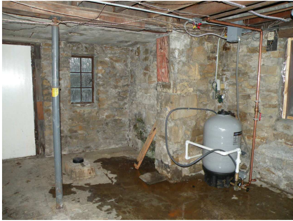
Water softener has been relocated
