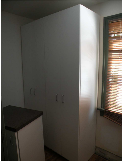
Work area cabinets
