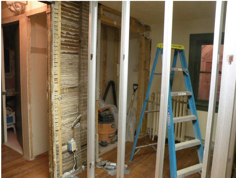
From former closet to new office space-closets have been removed and the new walls are in place.
